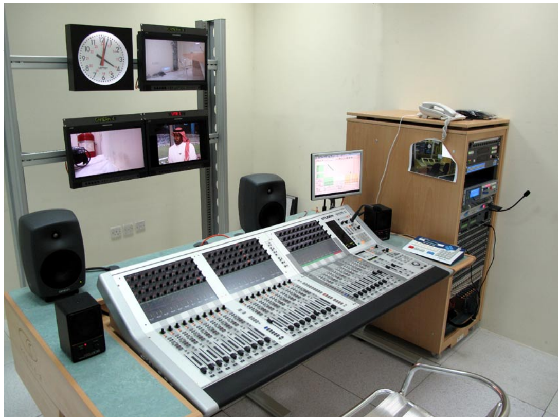
Apparatus racks and audio control suite
